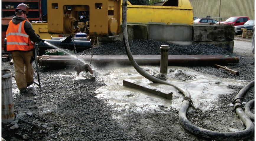
Photo B-5. Grout returned to ground surface at completion of Pile 5 installation.
