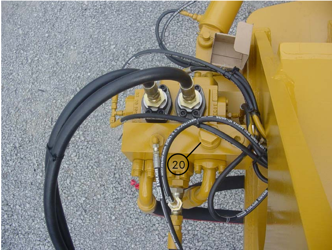
PHOTO 9: LEFT HAND SIDE SHOWING WINCH MANIFOLD
